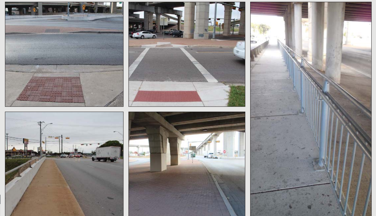
Figs A.8-A.12 Pedestrian Facilities Include ADA Ramps, Crosswalks, Sidewalks, and Hardscape Paving (clockwise from upper left)
